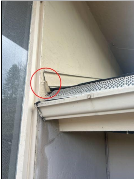
7. Kickout flashing - missing
