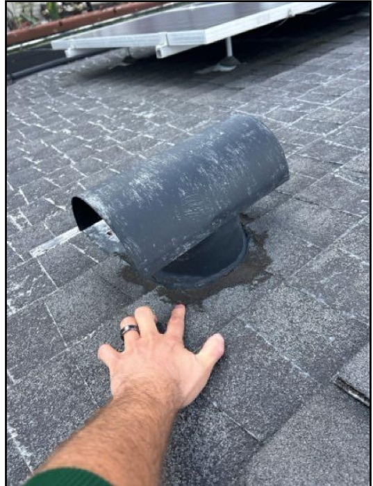
10. caulking has deteriorated
