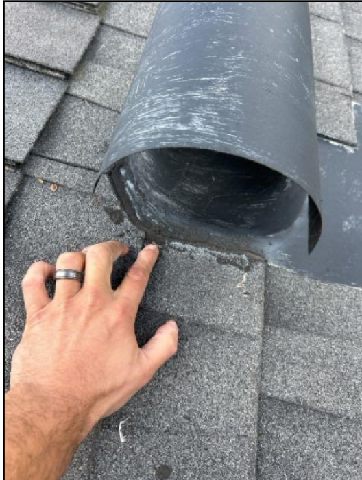
9. caulking has deteriorated
