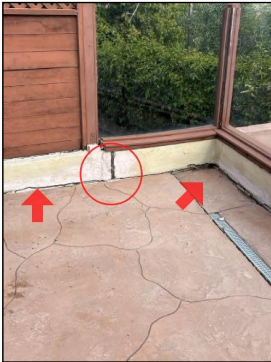
26. Crackes and slopping away
