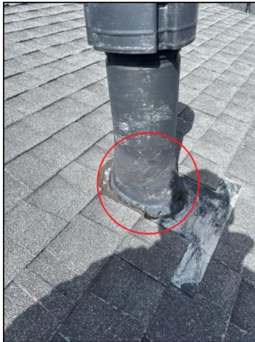
11. caulking has deteriorated
