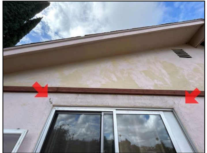
18. cracks at corner of door
