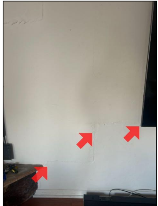
54. Second staggered cracked
