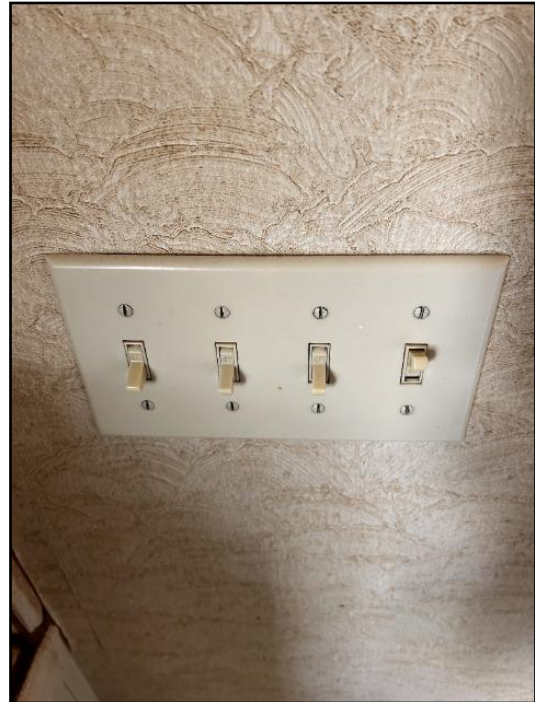
34. 3 left switches are Inoperative
