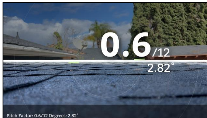
4. Slope too low
