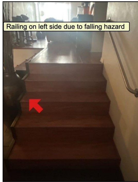
60. Railing needed on left for falling hazard
