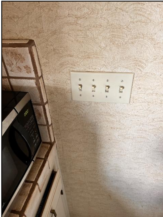
35. all switches turned on
