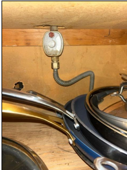
62. Gas shut off valve is not visible
