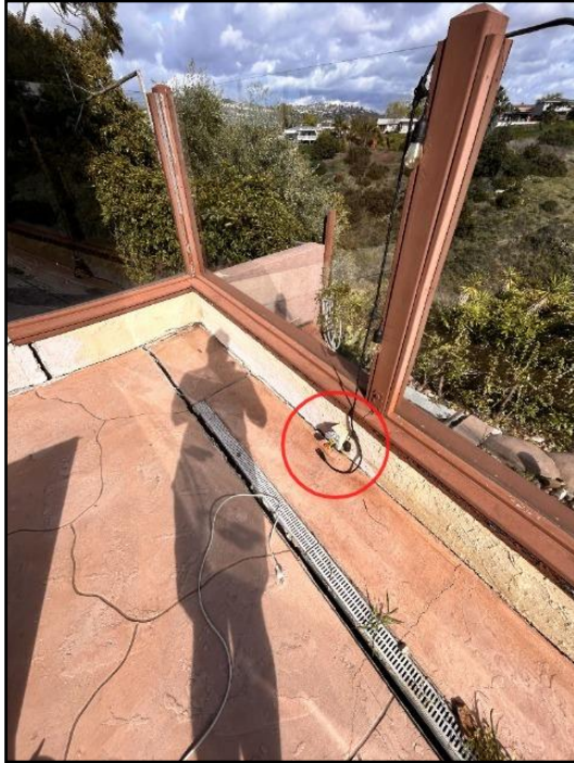
42. GFCI needed at exterior
