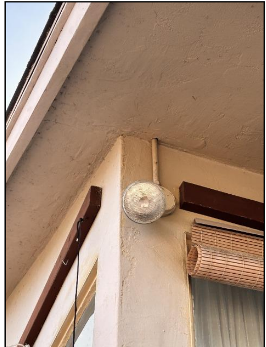
36. Flood light Inoperative
