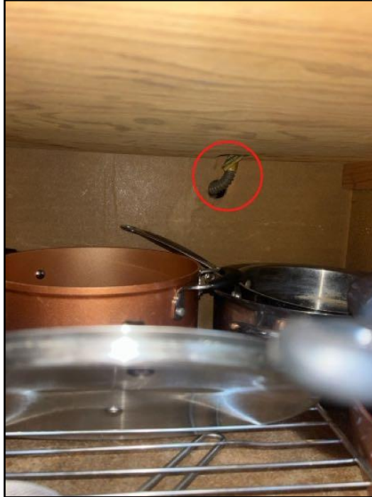
61. Gas connector passes through cabinet walls
