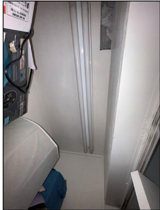
47. Improper closet lighting
