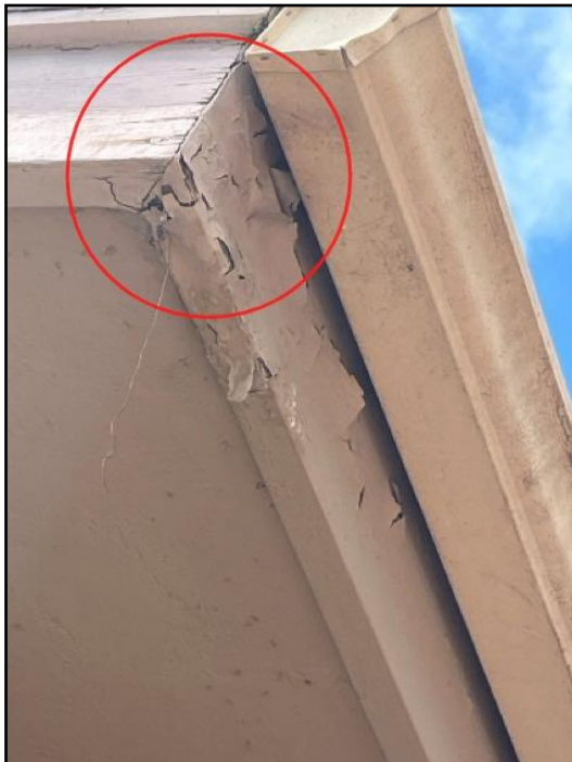
19. Paint has deteriorated will lead to rotten wood
