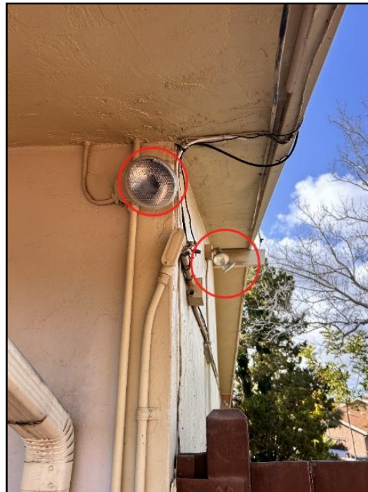
37. 2 flood lights Inoperative
