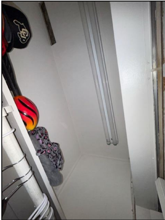
46. Improper closet lighting
