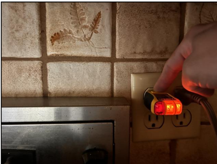
44. GFCI needed in kitchen
