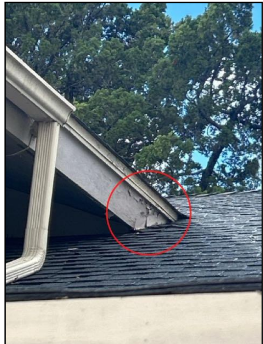
20. Paint deteriorated will lead to rotten wood
